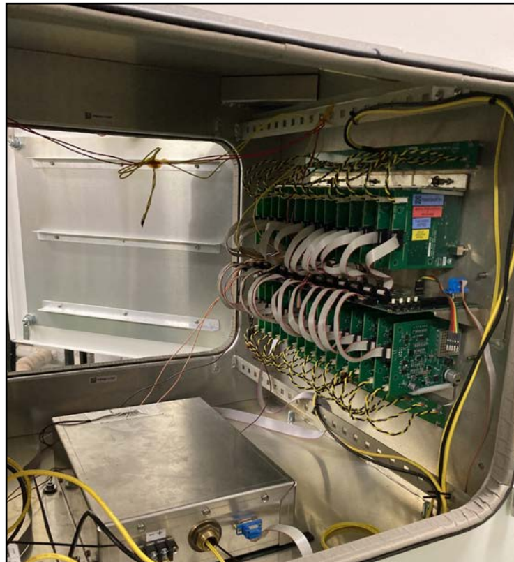
IMAGE ABOVE: Figure 2 The electronics Inside one of our prototype Field Node Distribution Hubs, built as part of the PaSD Project. Visible are 28 Power and Data over Coax Cards (PDOC's), 2 48v Power Distribution boards and the Field Node Control Board. The enclosure at the bottom of the image houses the FNDH communication equipment. Securing the parts for even this one prototype was a significant effort. IMAGE CREDIT: David Emrich
