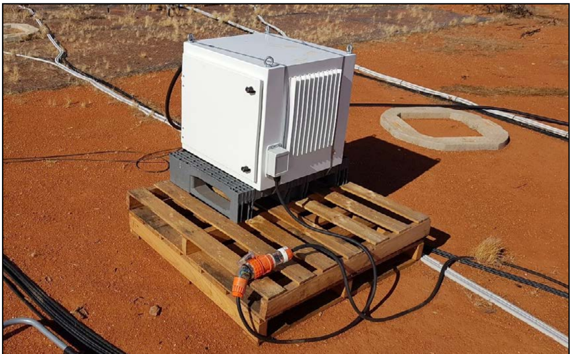
IMAGE ABOVE: Figure 2: Prototype FNDH on site IMAGE CREDITS: David Minchin
