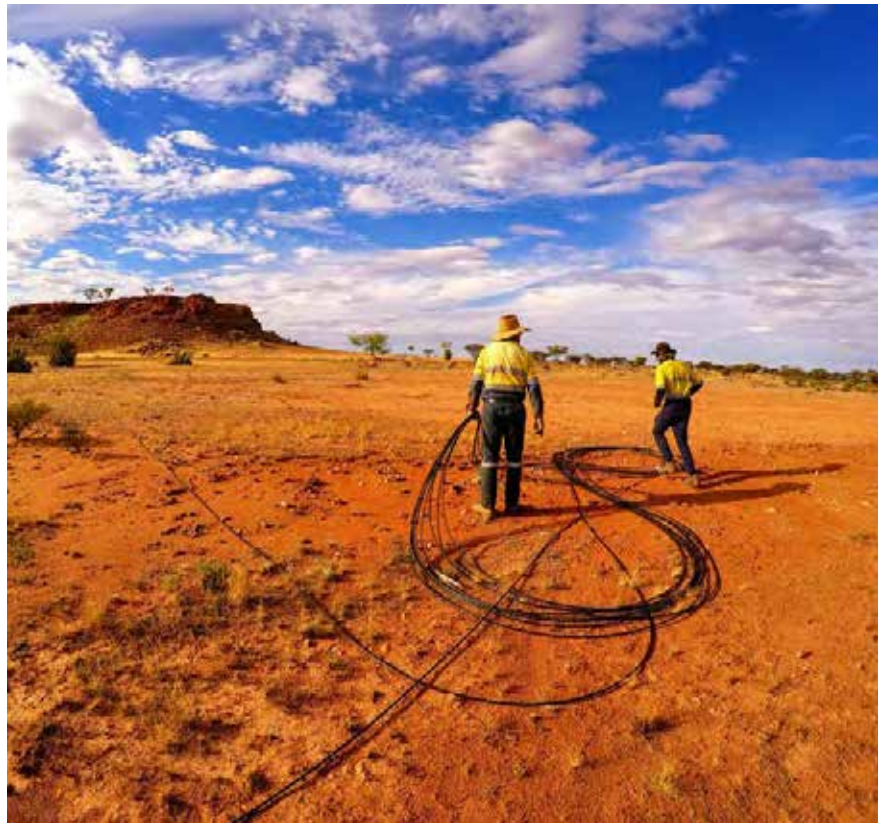
Wide angle view of GCo Electric running long (up to 2.6km) fibre cables out to distribution points, for the MWA Long Baseline tiles. Image Credit: Curtin University
