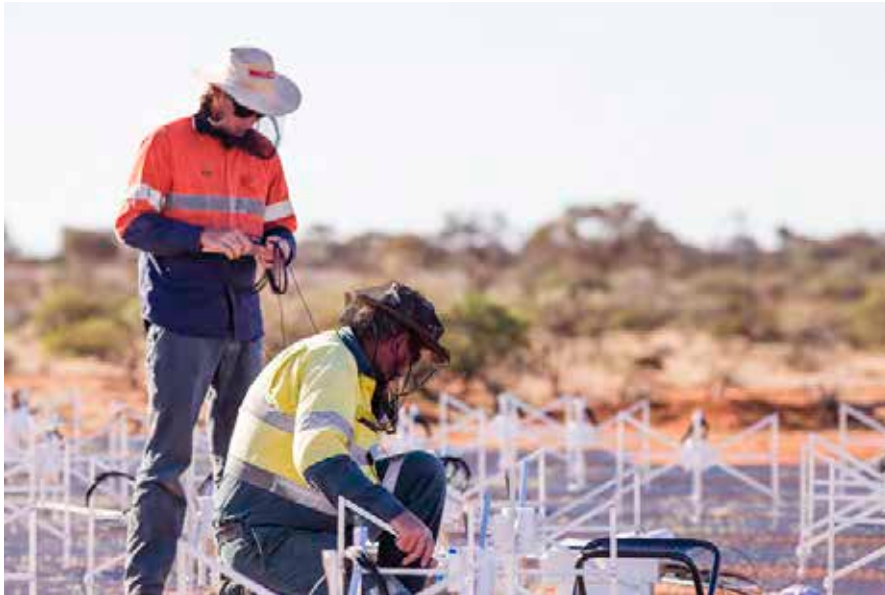
Figure 7, left: GCo Electrical contractors connecting cables between EDA2 antennas and SMART boxes. Credit: ICRAR, 2019
