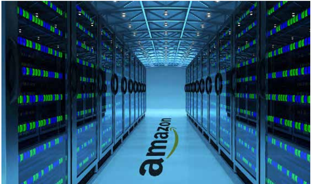
Figure 1, above: An example of the racks of equipment at Amazon Web Services (AWS). Credit: Amazon
